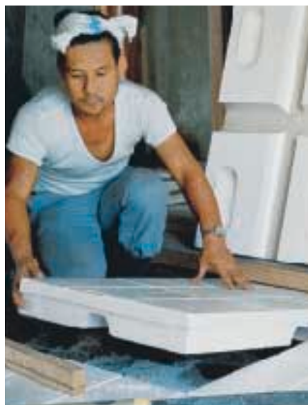
Fig. 23: Laying moulded Styropor elements for the thermal insulation of the normal floor construction in Japan
